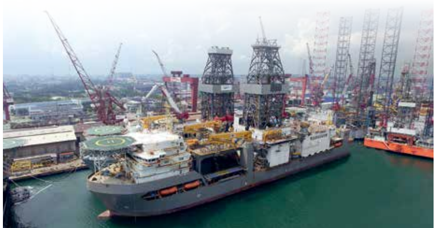
With immaculate planning from the project team, heavy lift installations for the topside modules have been executed like clockwork on the CAN DO drillship
